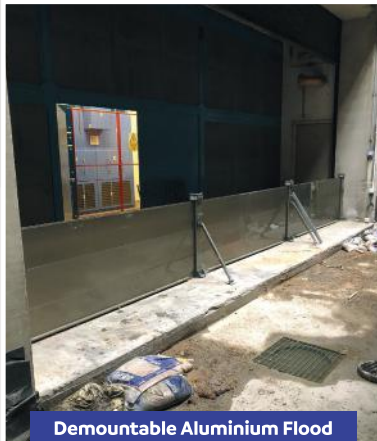
Demountable Aluminium Flood Barrier to Roller Shutter
