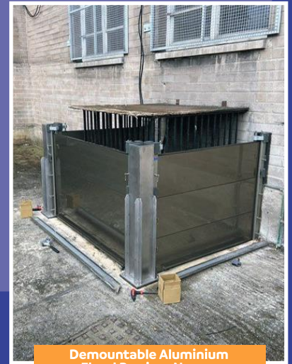
Demountable Aluminium Flood Barrier - Newry
